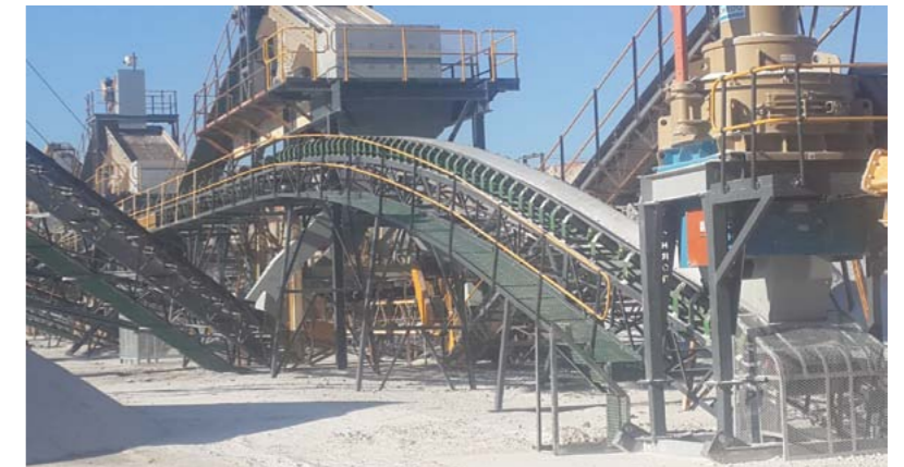
Curved Conveyer being implemented at Denver Quarry
