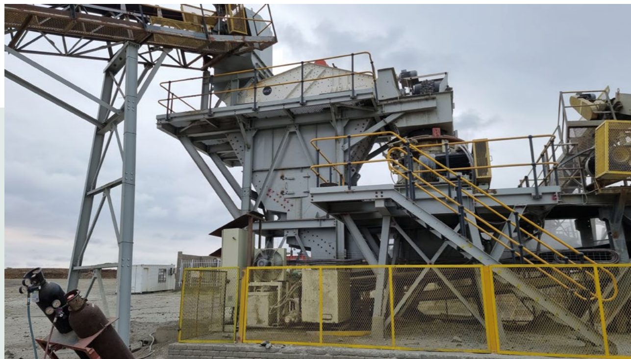
The plant after upgrading
