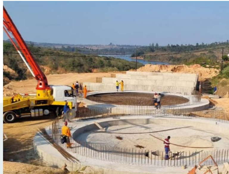
Maviljan Wastewater Treatment Works in Bushbuckridge
