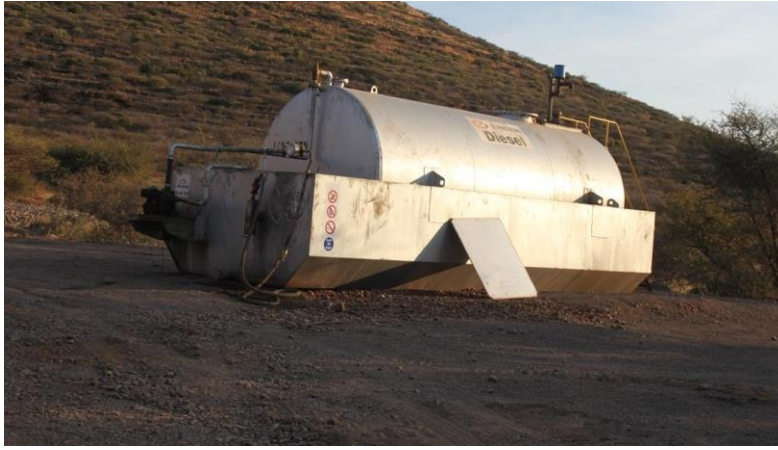
Photo 11: Steel bunded diesel tank of less than 30 000L
